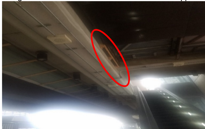
Figure 2: Previous Location of Steel Bracket Support
