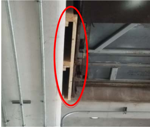
Figure 6: Incident 1 Temporary Repair
