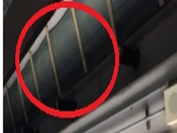
Figure 7: Incident 2 Safety Netting
