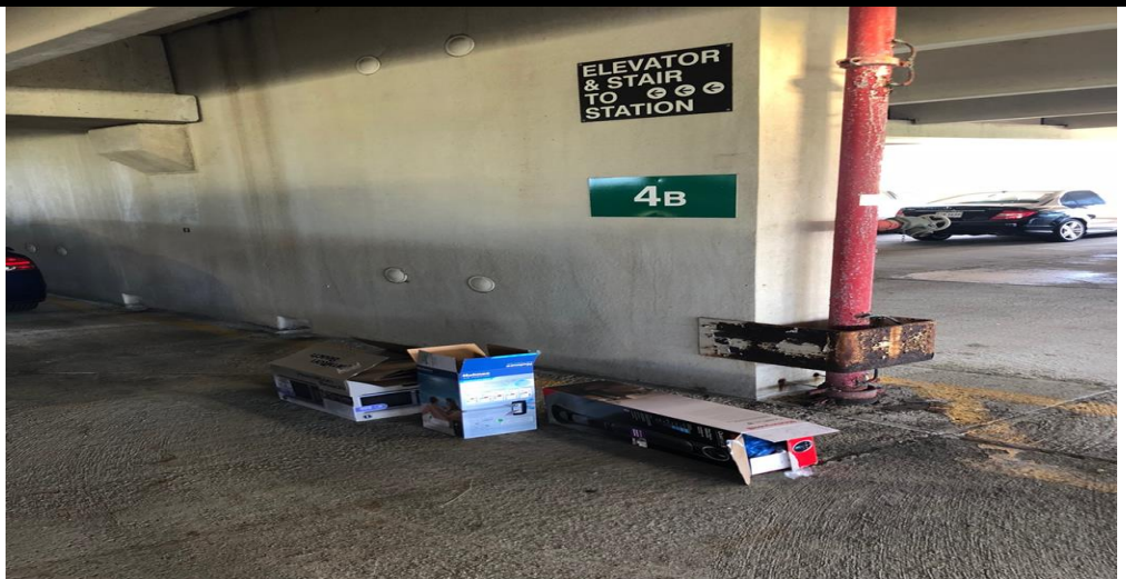
Date: June 11, 2019 Source: OIG
